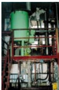
The CFB pilot plant
