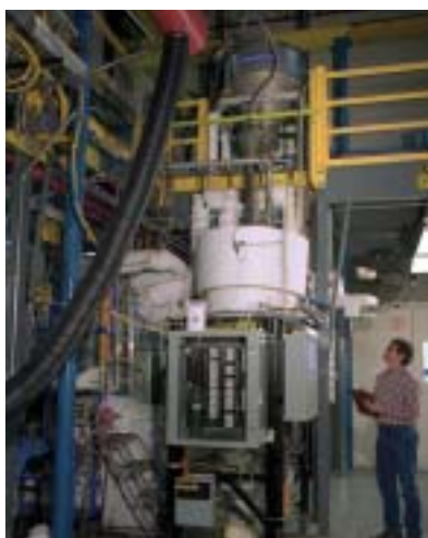
Figure 2: 20kg/h Fluidized Bed Reactor.
