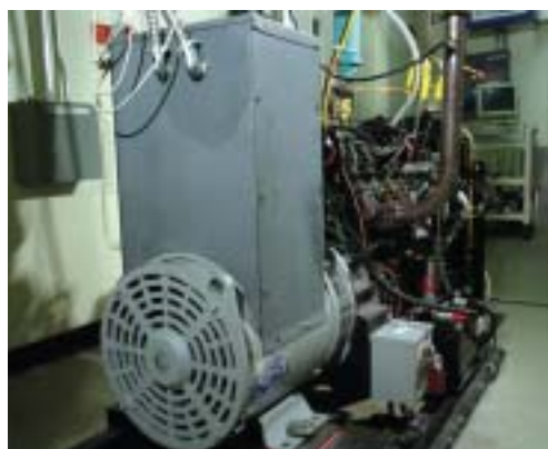
Figure 3: 15 kW Ford Engine Generator.
