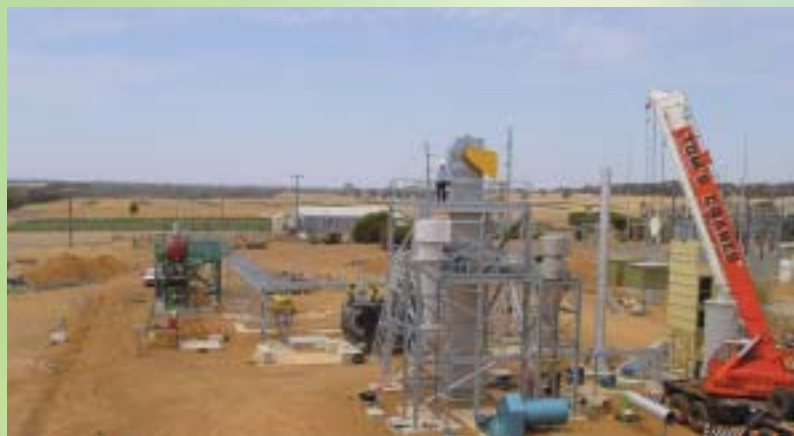
Figure 1: Construction work on demonstration plant in WA, February 2003. Photo courtesy of Western Power Corporation.
