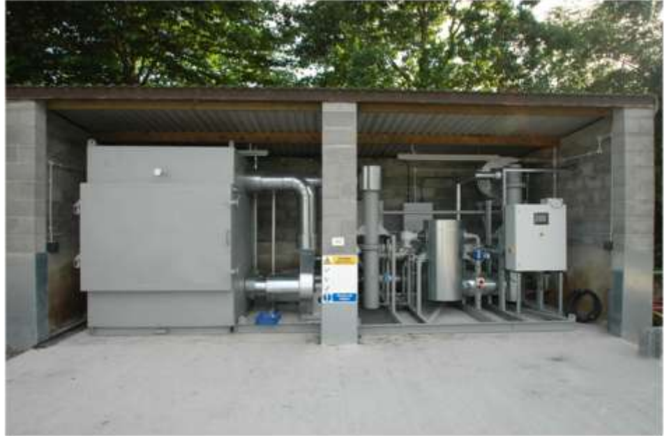
Figure 1: 500 kg batch slow pyrolysis reactor installed on site at IBERS, Aberystwyth.
