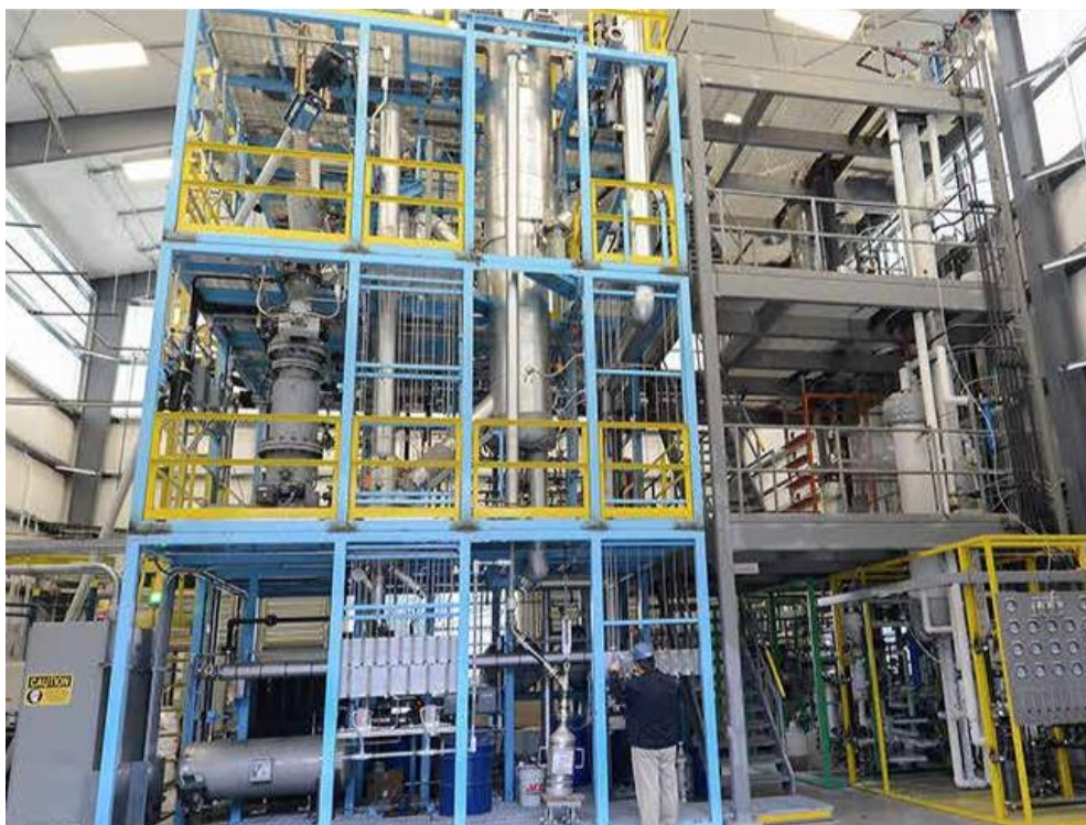
Fast pyrolysis pilot plant at RTI International in Research Triangle, North Carolina. The plant has a capacity of 1 tonne of dry biomass per day.
