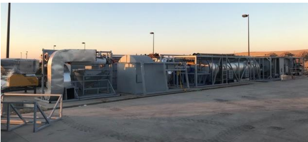
Biogas Energy Ltd.'s ablative fast pyrolysis pilot plant modules at an organics recycling facility in Placer County, California. The technology and reactors were provided by thermophil international.
