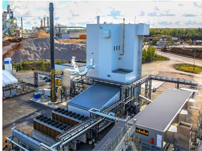
Picture of the Pyrocell pyrolysis plant in Gävle, Sweden.
