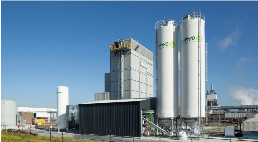
Fig. 5 A : Silos for storing wood crumbles; volume is 2x200 m 3 sufficient for 2 days.
