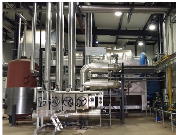
Fig. 8 B : Photo of the boiler
