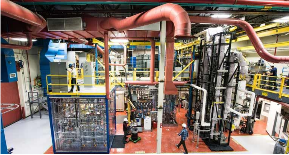
The Thermal and Catalytic PDU at NREL in Golden, Colorado.
