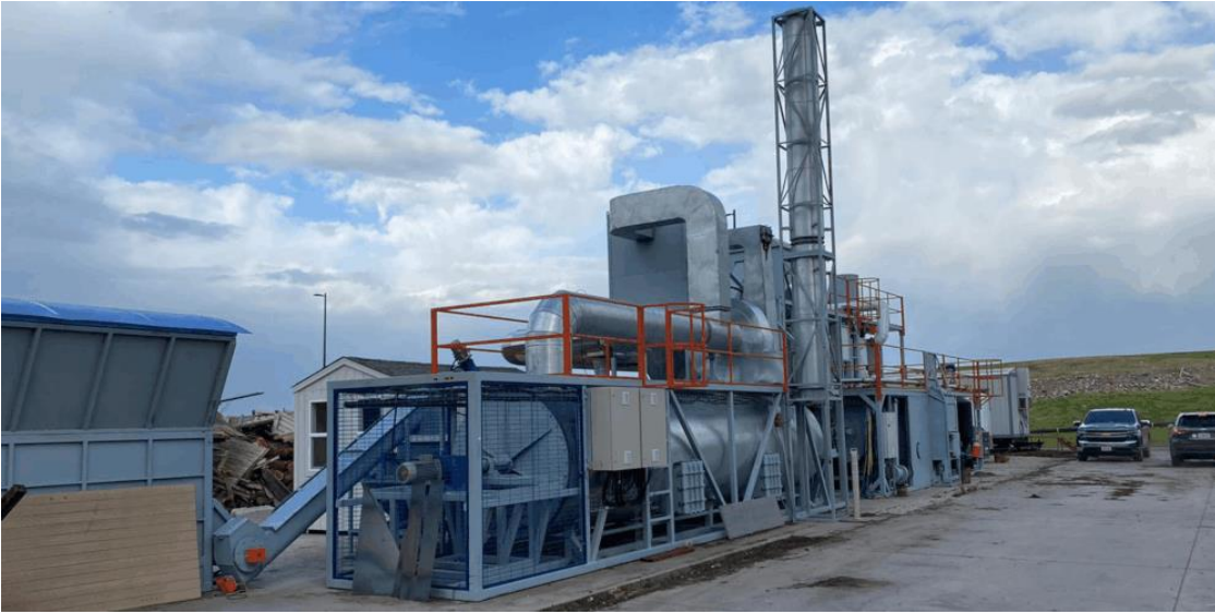
Biogas Energy Ltd.'s ablative fast pyrolysis pilot plant modules at an organics recycling facility in Placer County, California. The technology and reactors were provided by thermophil international.
